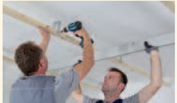
Aligning the laths with a spirit level or laser level and fastening of the lath to the hanger with two screws each per side.
